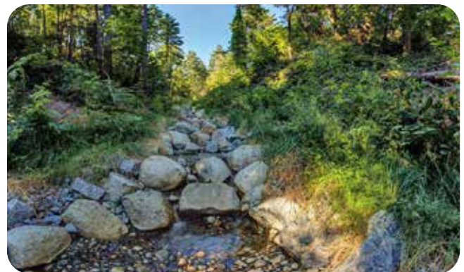
Stabilization project on steep slopes along John Matthews Creek. Photo credit: Burnaby Now
